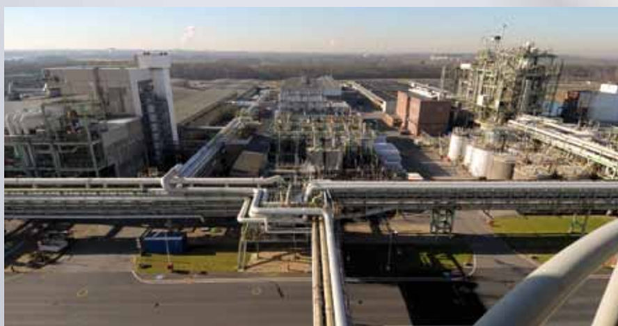
Baypren production plant in Dormagen/Germany. Photo Lanxess AG
